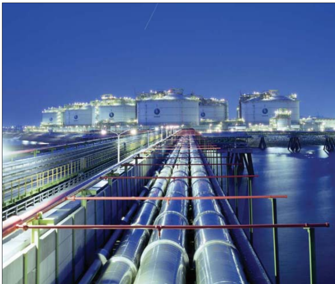
Korea Gas Corp. operates three LNG import terminals, the one at Incheon (shown here) being the oldest, starting up in 1996. At Incheon, 18 tanks can store nearly 2.5 million cu m of LNG. Data for 2007, the most recent available, show that South Korea ranked second in total LNG imports behind Japan. Korea Gas is set to receive the first cargoes from Sakhalin 2 in second-quarter 2009. (Photograph from Kogas)
